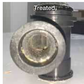
Water heater outlet
